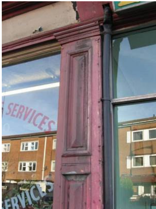
Some of the shopfronts have been partially removed but retain tantalising glimpses of the original shopfront.
