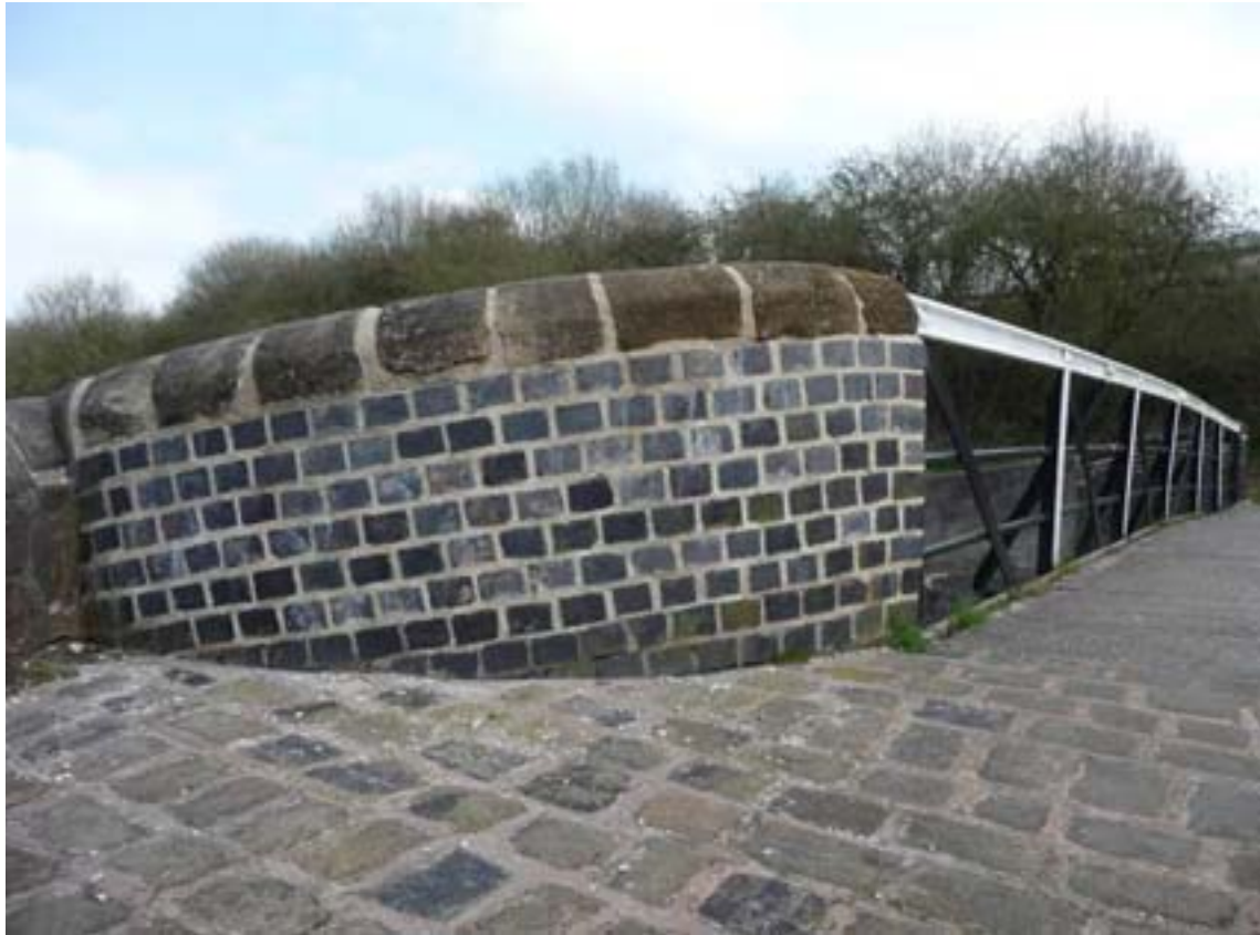
Fig. 5: Header bond and stone copers to brickwork in Bridge 130, with traditionally designed stone setts and metal railings
