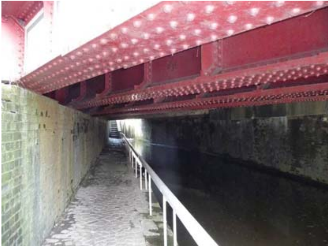
Fig. 42: Railway bridge cuts across the canal south of Cockshott Lock, creating a strong sense of enclosure
